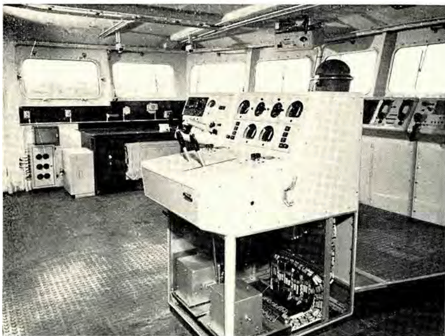
Steering and machinery control console as fitted on the bridge of the Mark 5 frigate
